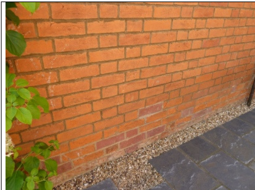
High ground levels against the right hand flank wall.
