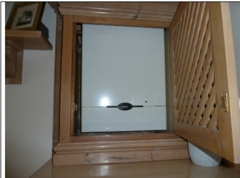
Baxi boiler in the kitchen.
