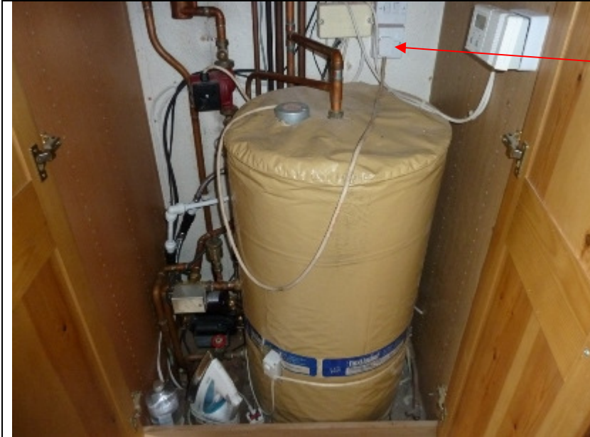
Hot water cylinder. Note the immersion heater is wired to a 13 Amp plug.
