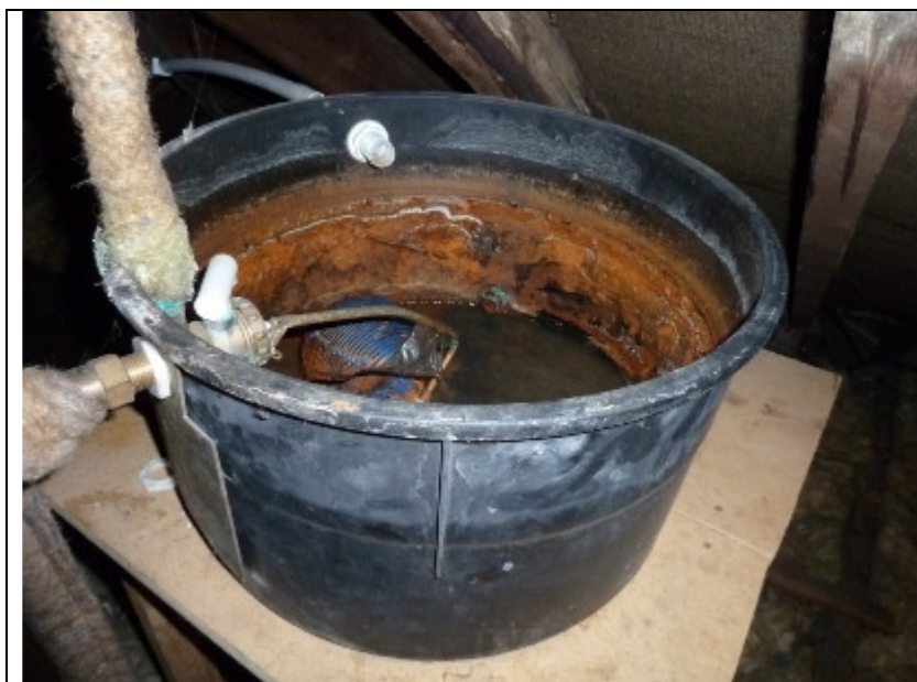
Feed and expansion tank in the roof space.
