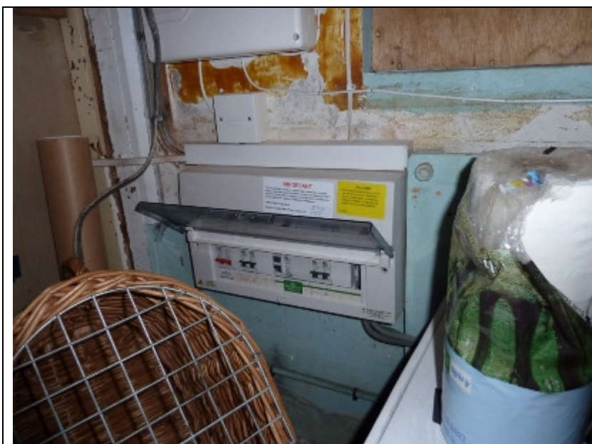
The consumer unit in the under stair cupboard.
